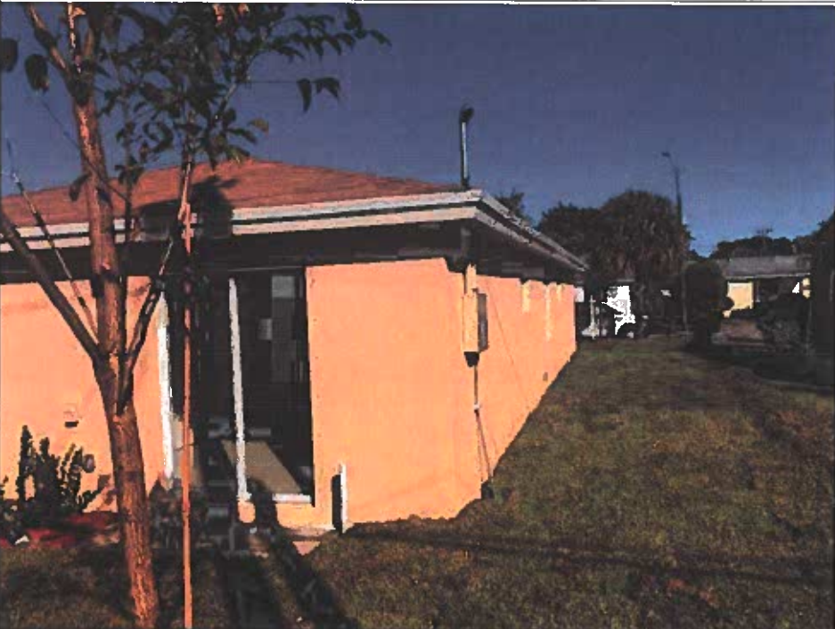
Photo Two Caption LEFT VIEW (01/21/2020)
